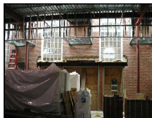
The new entrance to the chapel with the skylights over the windows
